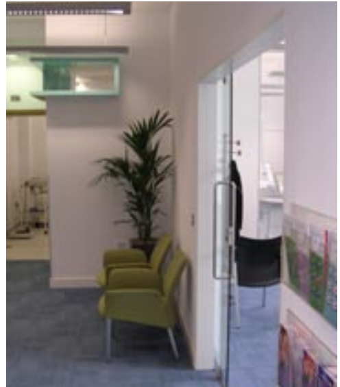
Carefully detailed high level glazing throughout the health centre provides natural light and also ensures privacy
